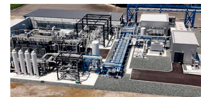
Chita-Midorihamas Works Hydrogen Production Plant (Commenced operations in June 2024)
