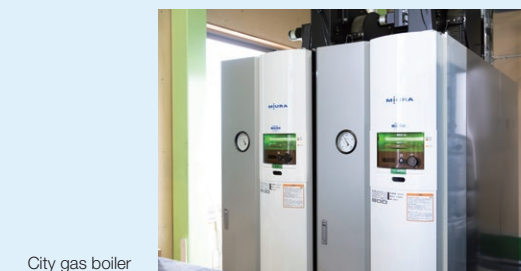
City gas boiler
