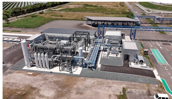
Hydrogen production plant at Chita-Midorihama Works
