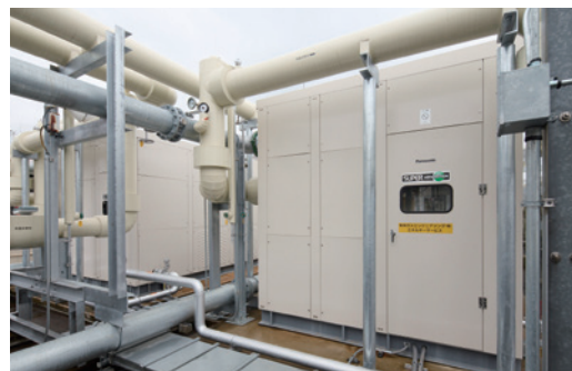
Two highly efficient, natural chiller units
