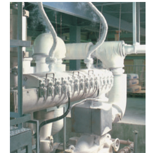
Low-temperature grinding plant
