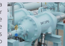
Electrical power turbine generator
